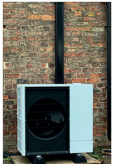
THIS INSTALLATION HAS PROTECTED THE PIPEWORK AND INSULATION IN EXTERNAL GRADE TRUNKING. NOT ONLY DOES THIS OFFER EXCELLENT LONG-TERM PROTECTION BUT LOOKS MORE AESTHETIC AND GIVES THE INSTALL A FINISHED LOOK.
