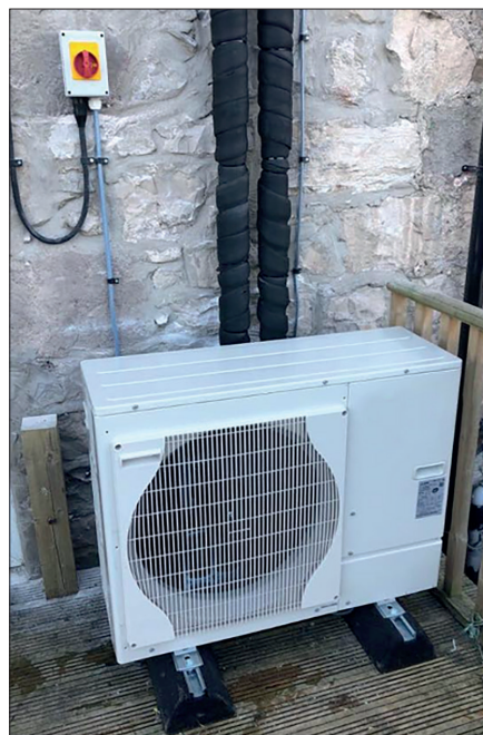
THE INSULATION SHOWN IS WRAPPED AND INCONSISTENT IN THICKNESS DUE TO THE TIE WRAPS - THUS REDUCING THE INSULATION QUALITY.
