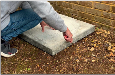
STEP 1 - Position and mark ground for the required location of the FLEXI Lite Slab.
