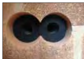
3. INSERT THE PVC SLEEVE INSULATION, RECESS IT TO ALLOW FOR THE ELBOW TO BE LOCATED.
