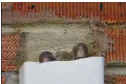
THE CONNECTION OF THE PIPEWORK RUNNING THROUGH THE WALL
